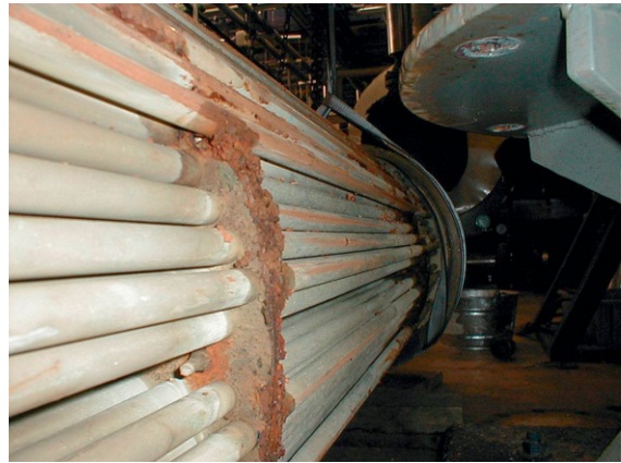
Photo 4 Scaled and corroded condenser tubes.
