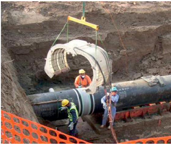
Figure 5 An induction coil being lowered into place over a prepared field joint on a large diameter pipe.
