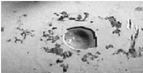
Figure 3 Typical AC corrosion on an fusion bound epoxy-coated pipeline. Reproduced from AC Induced Corrosion on Onshore Pipelines, A Case History, Roger Ellis Shell UK, Stanlow, 2001. Pipeline Manager UKOPA (United Kingdom Onshore Pipeline Operators' Association).
