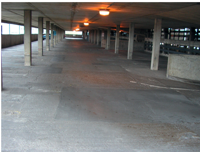
Figure 5 Multiple patch repairs to car park deck.
