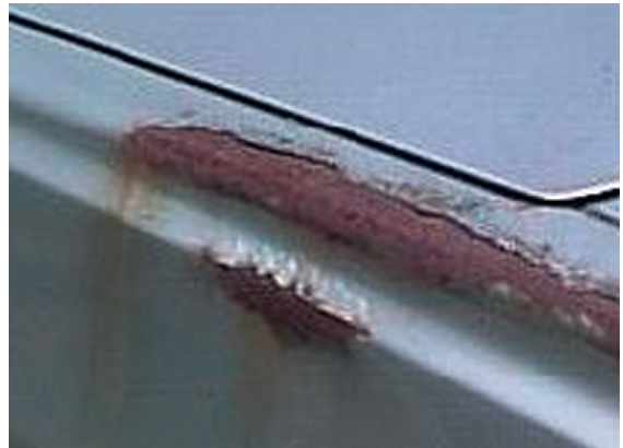
Figure 2 Corrosion along a panel bend.
