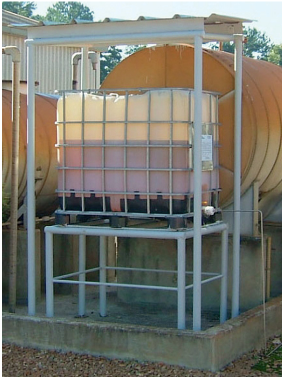
Photo 12 Chemical corrosion inhibitor feeding station.
