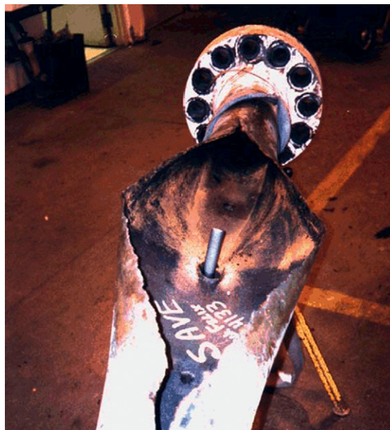
Figure 7 Failure of line at injection point. Corrosion Threats Handbook – Upstream Oil and Gas Production ; Energy Institute of Oil and Gas: London, 2008.
