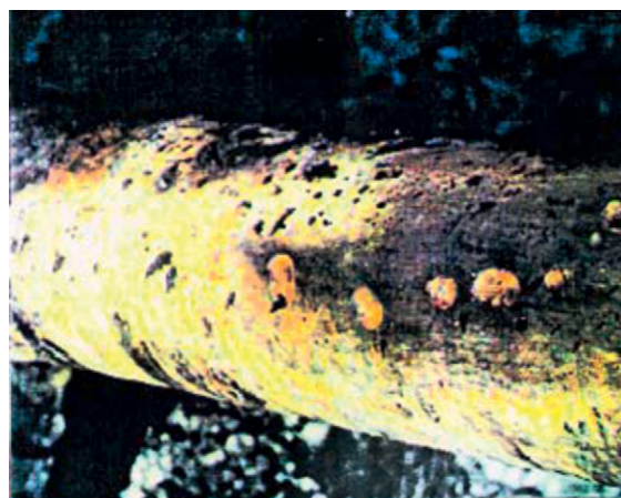
Figure 2 Typical AC corrosion on a bituminous-coated pipeline. Reproduced from Corrosion due to AC on metallic buried pipelines: Background and perspectives L. Di Biase APCE, 2nd National Conference, Rome, Nov. 1996; pp 21–22.
