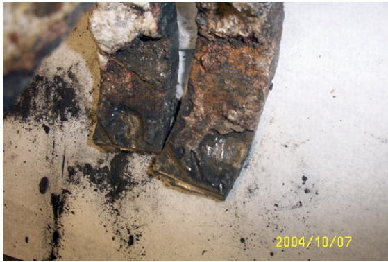
Photo 5 Oxygen pitting corrosion.
