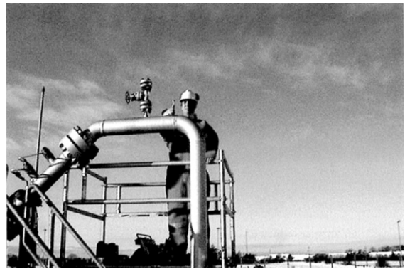
Figure 9 Field Signature Method (FSM) – Installation on piping at bend/weld on piping (Courtesy iicorr Ltd.).
