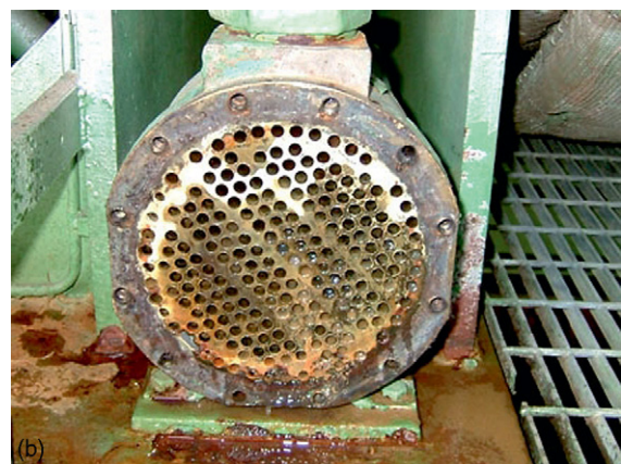
Photo 7 (a) Algal fouling on a cooling tower and (b) fouled and corroded heat exchanger.
