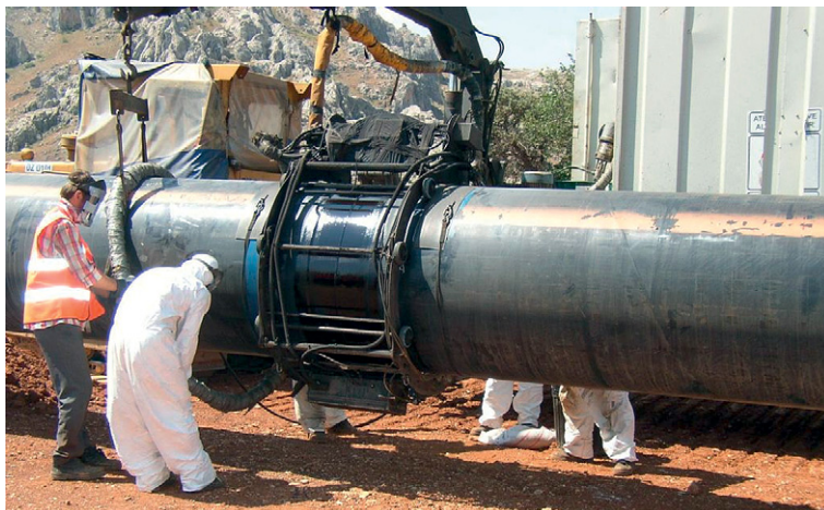
Figure 4 Application of a two-pack solvent-free liquid coating to field joints on large diameter pipe.
