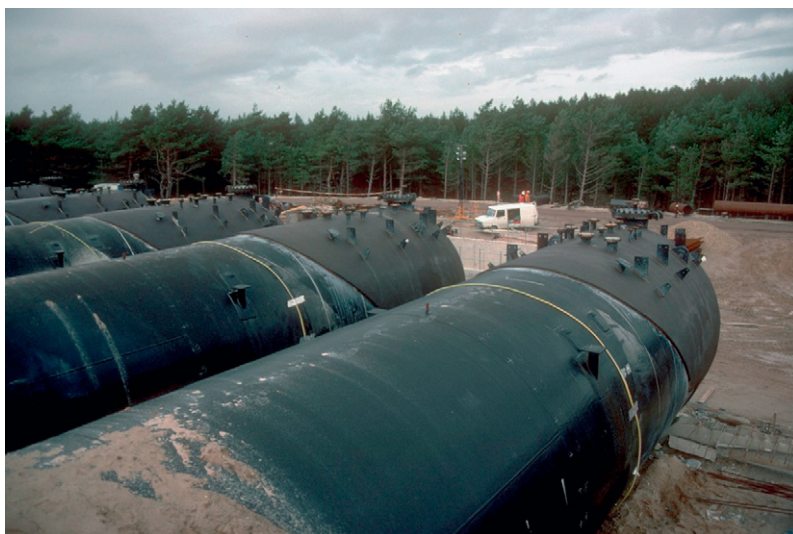
Figure 1 Large LPG storage tanks externally coated with a solvent-free coal tar urethane awaiting burial.
