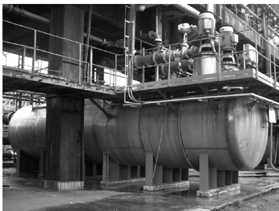
Figure 25 Anodically protected tank for storing pure sulfuric acid (94–99%) at temperatures up to 40 °C.
