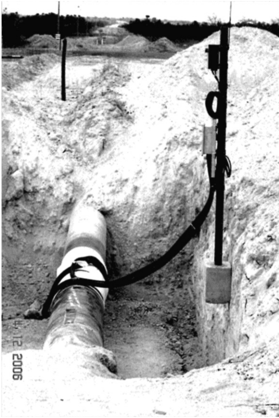
Figure 11 Field Signature Method (FSM) – Installation on buried pipeline (Courtesy iicorr Ltd.).
