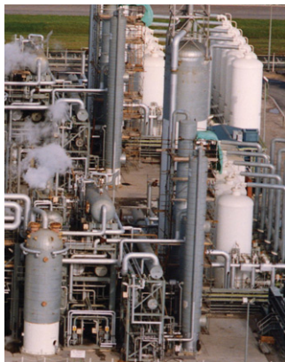
Figure 1 Process plants, regardless of size/complexity, are assembled from standard equipment items.
