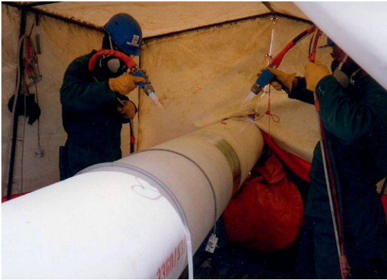
Figure 10 Flame spray application of polypropylene to pipeline field joints inside a weatherproof shelter.
