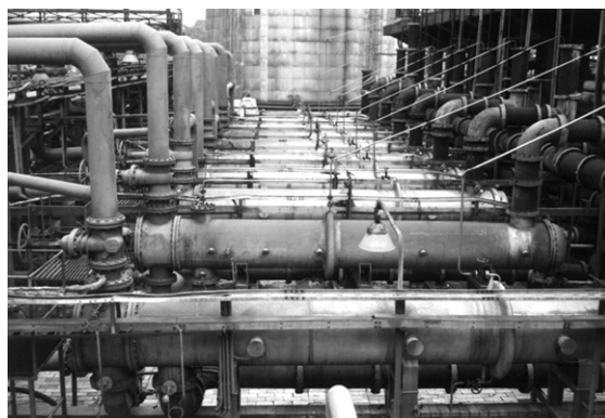
Figure 23 Anodically protected stainless steel heat exchangers for cooling of 93–98 wt% sulfuric acid.
