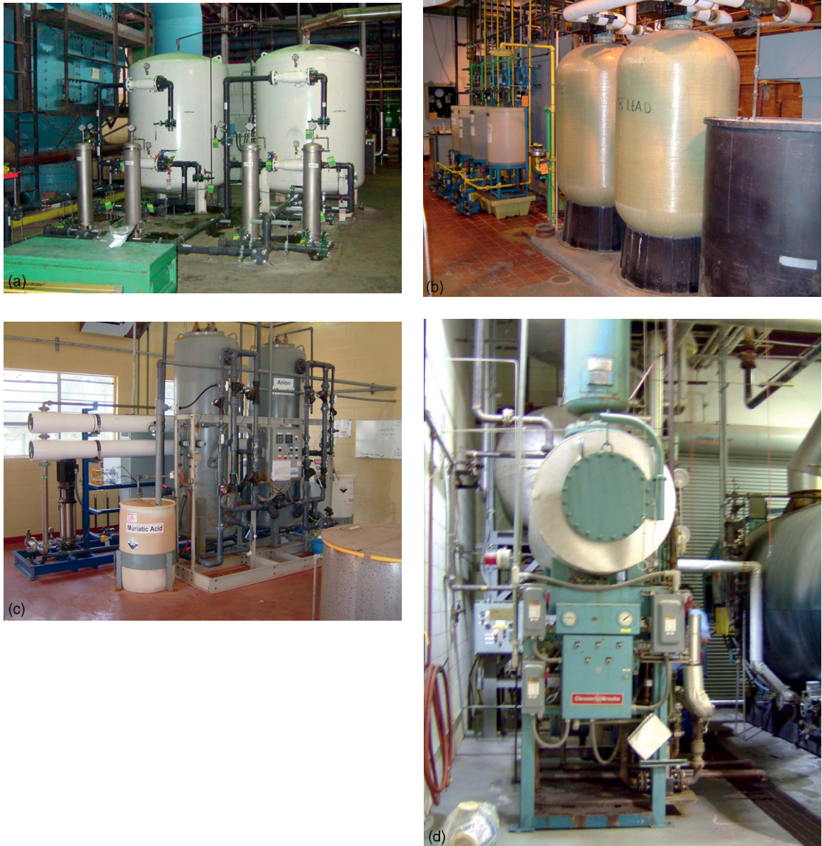
Photo 9 (a) Filters removing oil and organics from water, (b) twin ion-exchange water softeners with salt tank and chemical feed station, (c) demineralization and RO plant, (d) deaerator.
