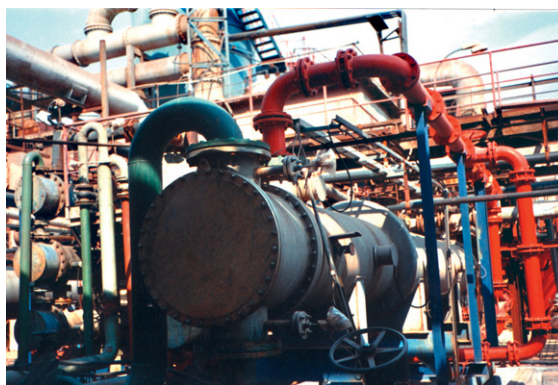
Figure 24 Anodically protected stainless steel heat exchangers for cooling of 75–78 wt% sulfuric acid.
