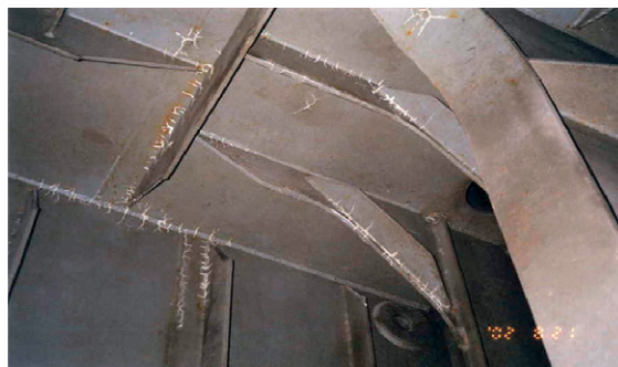
Figure 4 Cracking of coating in a ballast tank.
