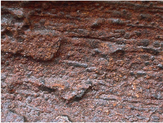
Figure 1 Erosion corrosion of a tubular (mesa corrosion).
