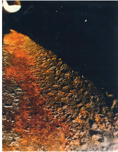
Figure 3 Pitting corrosion found under deposits in a pipeline.
